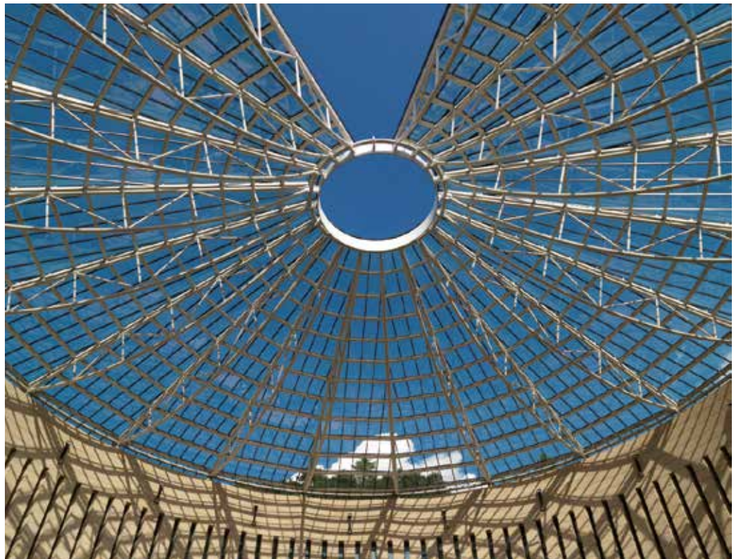
Museum of Modern and Contemporary Art of Trento and Rovereto, Italy / Structure to support the roof
